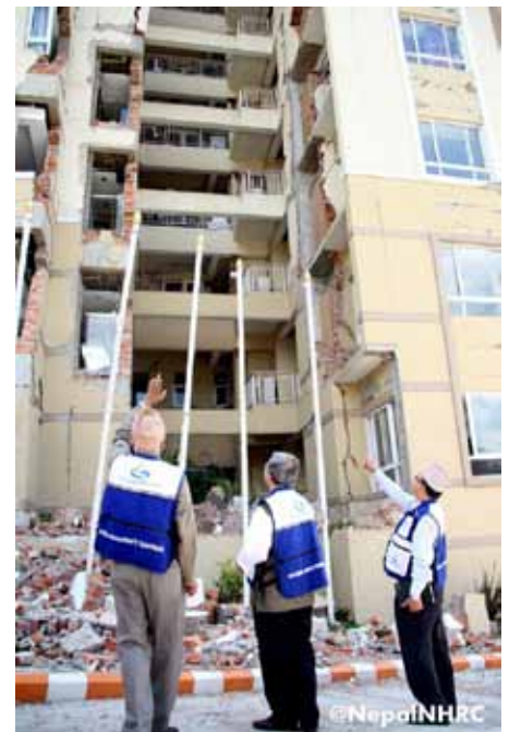
The NHRC high level monitoring team observing a highly damaged mansion in the valley during monitoring (Photo: Janak Raj Bhatta, Central Office)
