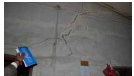
A crack seen on the wall of prison during the monitoring in Khotang district prison
