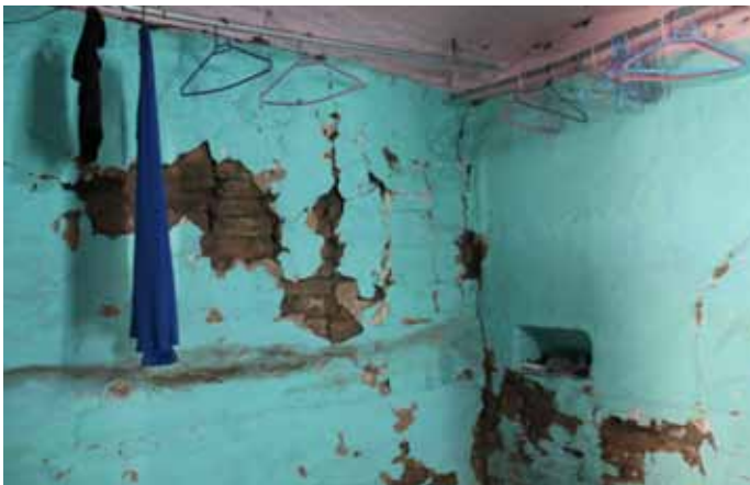
The damaged wall of the prison cell at the Central Jail, Kathmandu
